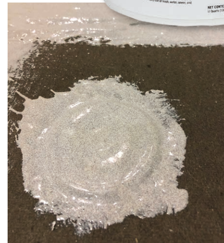
Acclaim® FSG applied by chip brush over fastener head, plate and seam on an impact resistant cover board system prior to coatings application.
