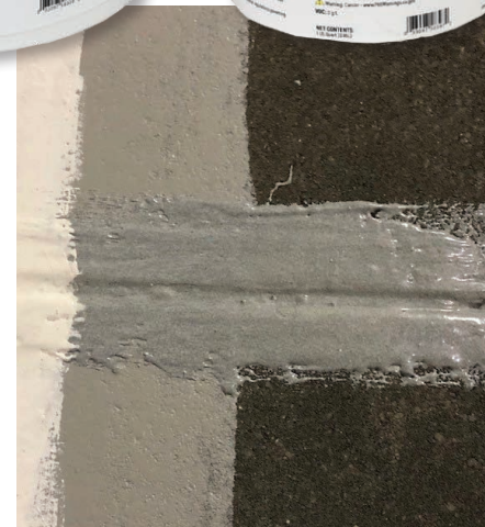
Acclaim® FSG applied by chip brush over seam on a concrete roof system prior to coatings application.
